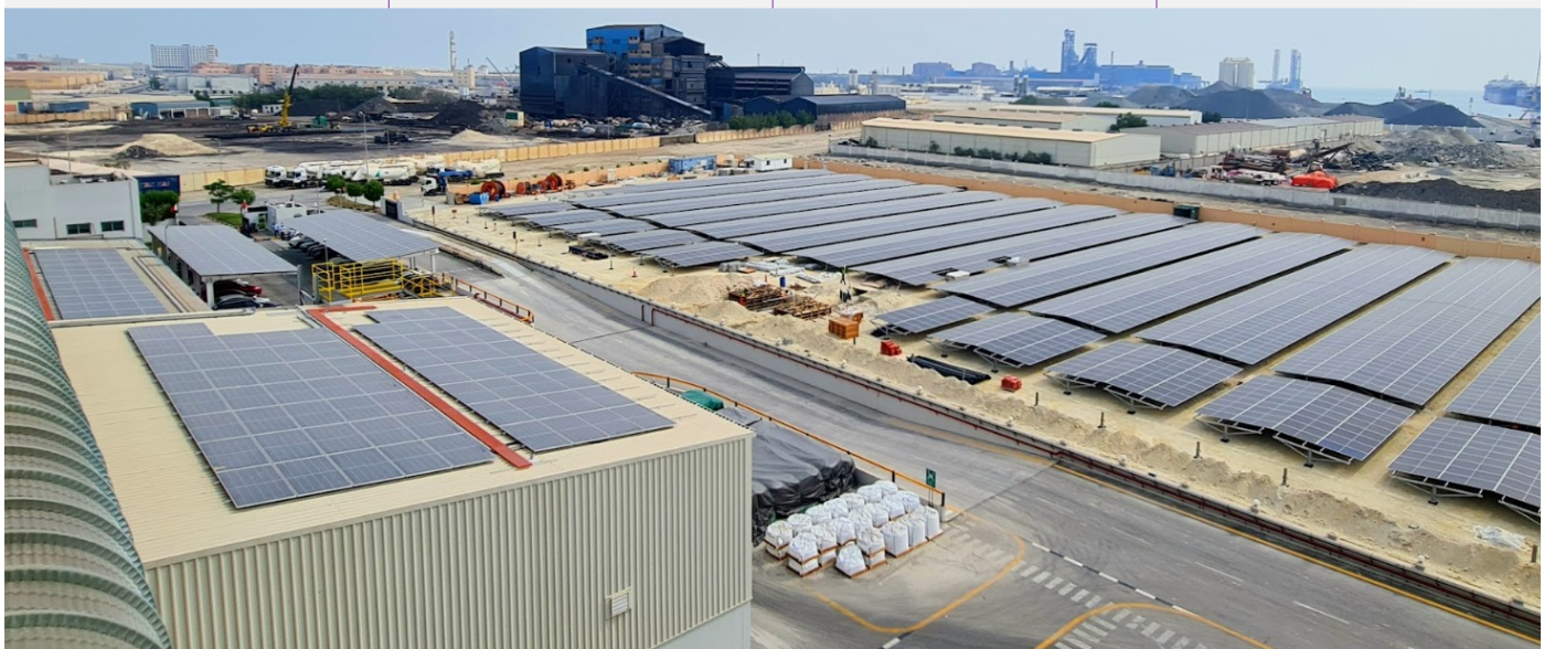
Hidd solar PV installation at our Al Zayani Fused Minerals site in Bahrain
